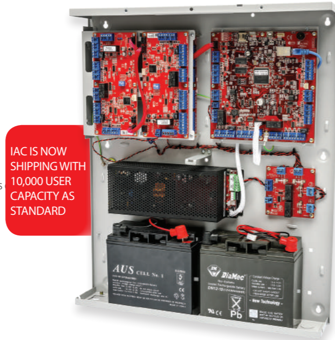
ABOVE: IAC shown in 8 Door / 10 Reader configuration. (IAC with UniBus 2 Door / 2 Reader expansion devices connected). Housed in the WideBody enclosure with hinge plate, 8Amp PSU, Fire Door override relay card and 2x 17Ah batteries
